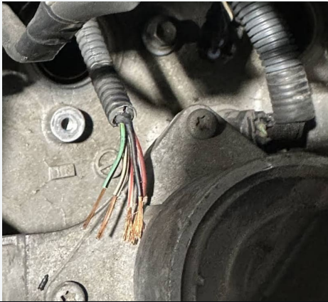
PHOTO 03 - Illustrative wiring concern (#91)
